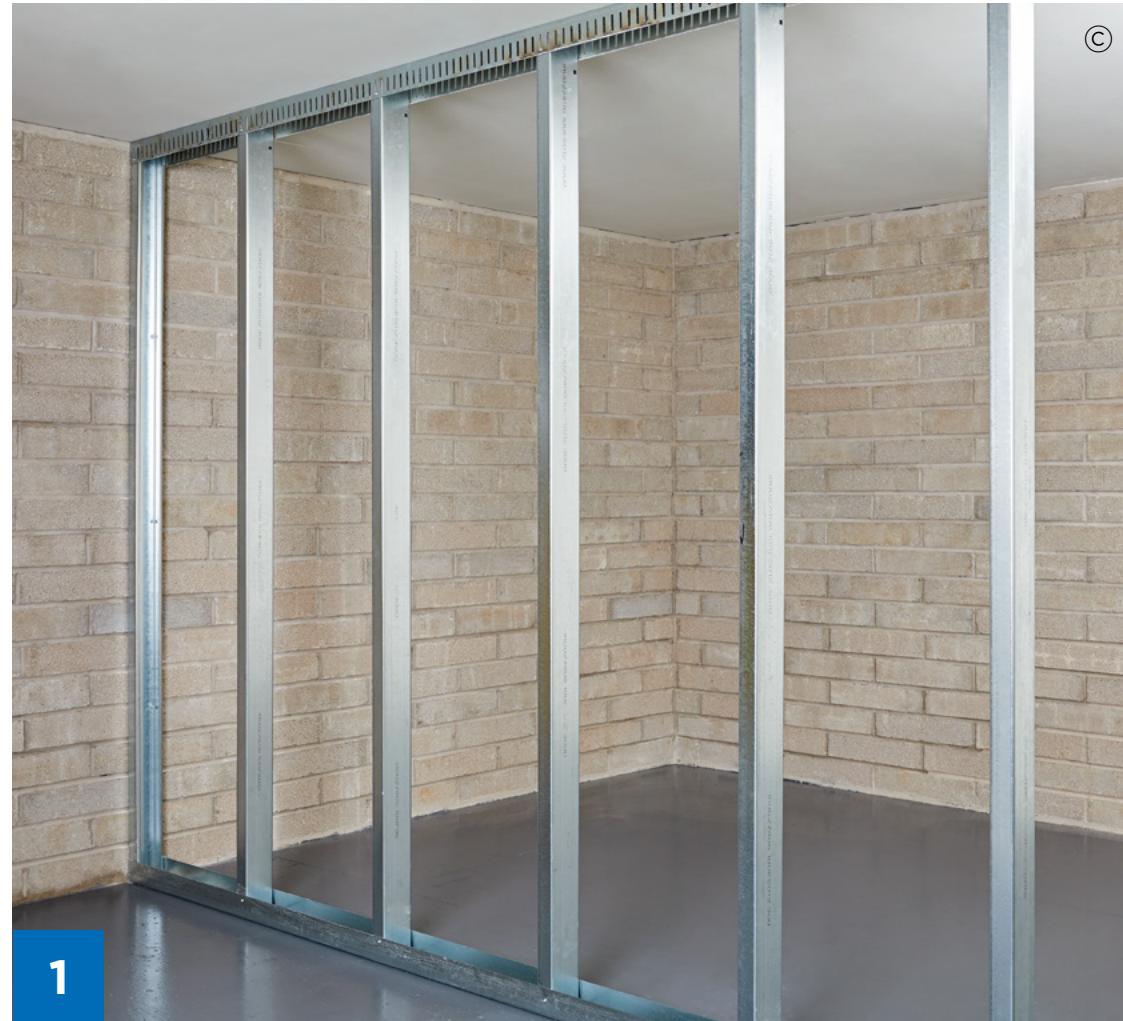
Completed Steel Frame System (SFS) framework ready to receive the Glasroc X Sheathing Board.
