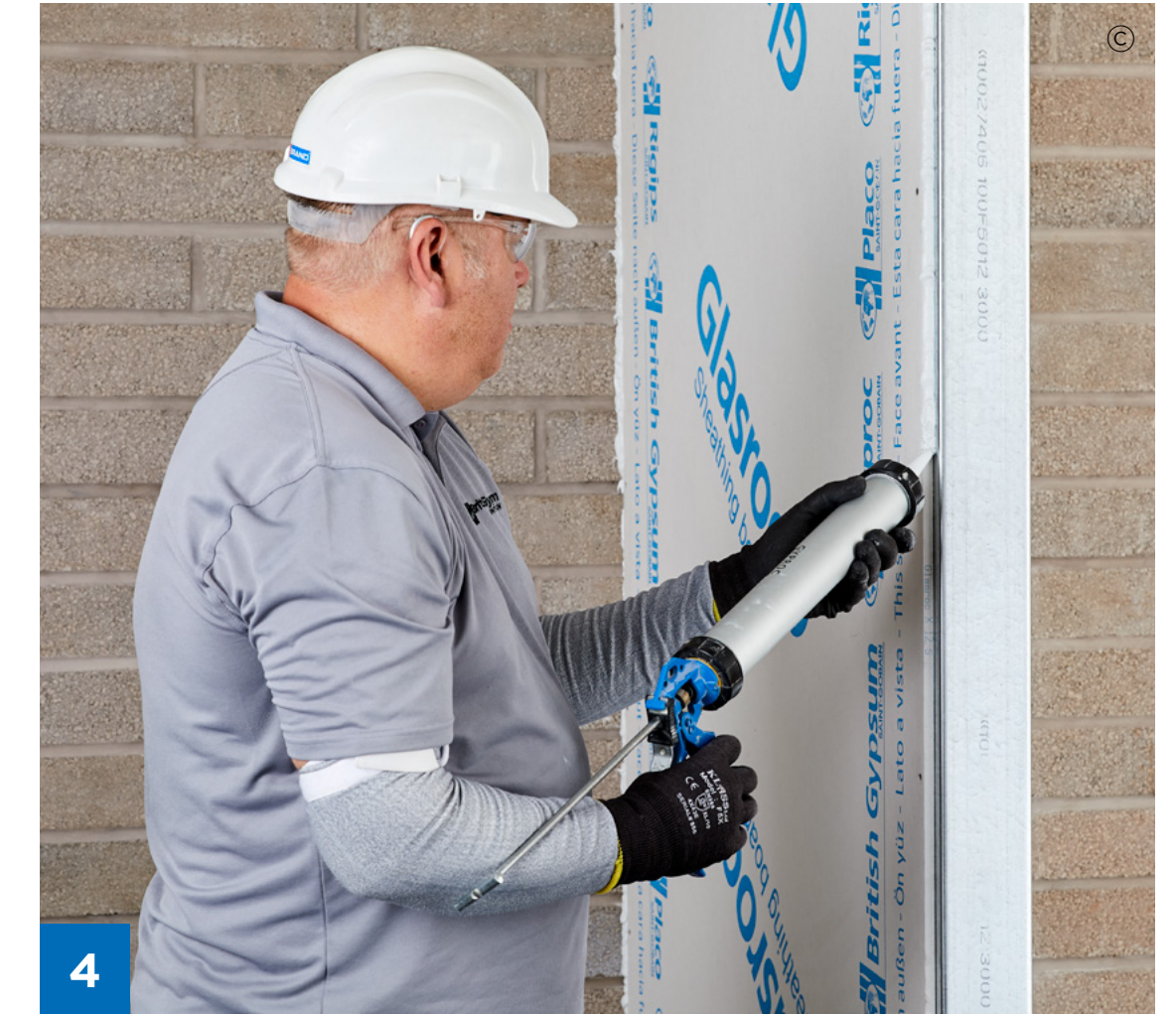
Run a continuous 6 mm wide bead of Glasroc X Sealant along the installed Glasroc X Sheathing Boards exposed edges, which will have other boards abutting against it.
