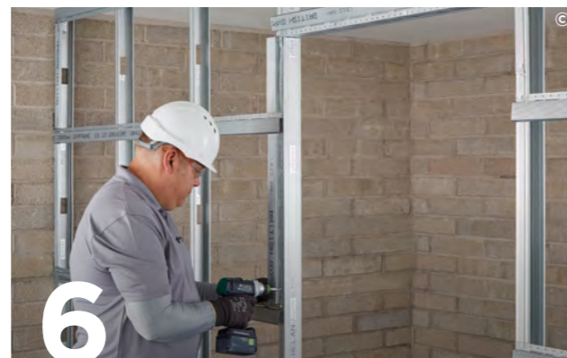
6 Install Gypframe RB1 Resilient Bars vertically to abutment and door studs to accept perimeter fixings for the Gyproc plasterboard linings.
