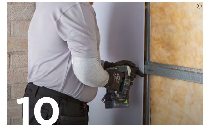
10 Use British Gypsum Drywall Screws to fix Gyproc plasterboards to the Gypframe RB1 Resilient Bars, with all joints staggered.
