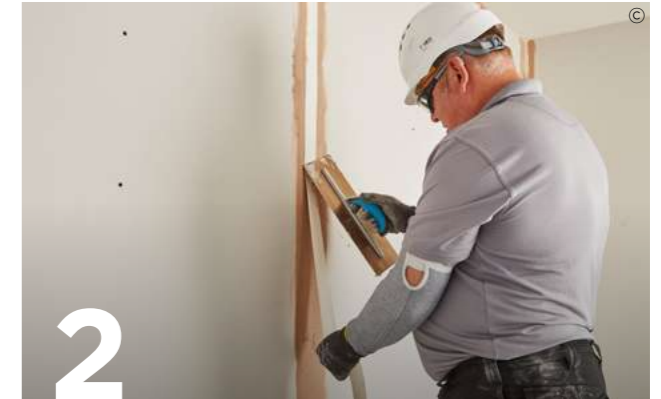
2 Where there is an increased risk of cracking, or where gaps exceed 3mm, the gaps are reinforced with Gyproc Joint Tape bedded in Thistle plaster. In other situations, plasterboard joints can be reinforced with Thistle ProTape FT50 or FT100 glass fibre mesh tape.
