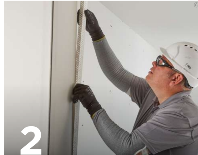
2 For external corners use the self-adhesive Gyproc AquaBead or Gyproc Corner Tape or Gyproc LevelLine which are bedded with a Gyproc setting compound.
