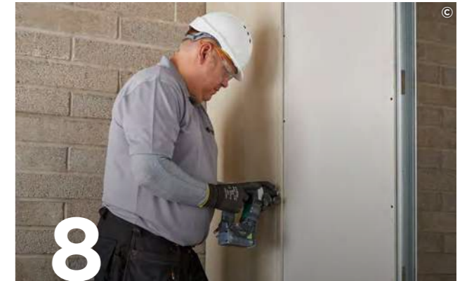
8 For an even more robust solution use Rigidur Screws to fix Rigidur H as the outer layer to all Gypframe framing members.
