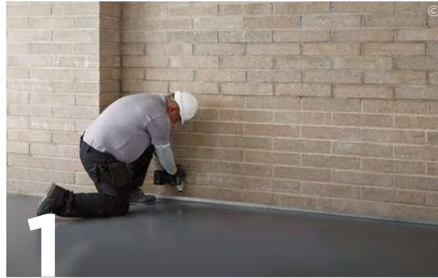
1 Suitably fix Gypframe GL8 Track to the perimeter walls at the required centres. Ensure the large lip faces internally.
