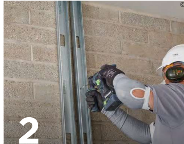
2 Fix Gypframe 'C' Studs to abutments and openings in two rows using suitable fixings.
