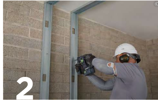
2 Fix Gypframe 92 S 10 'C' Studs at abutments and door openings in two rows using suitable fixings.
