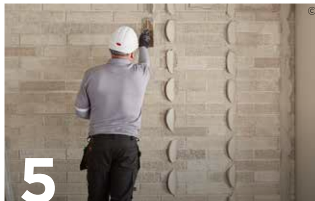
5 If using Gyproc DriWall Adhesive, apply methodically in a specific dab pattern to the appropriate background, ensuring 20% coverage is obtained.
