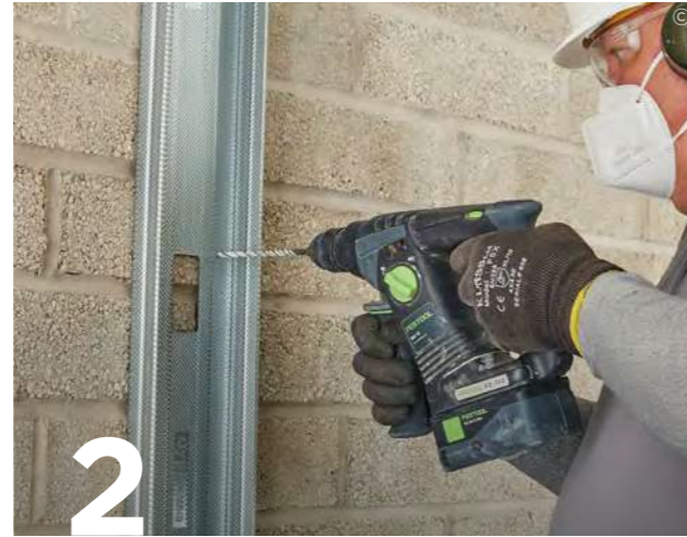
Fix Gypframe 'C' Studs at maximum 600 mm centres to abutments and openings using suitable fixings.
