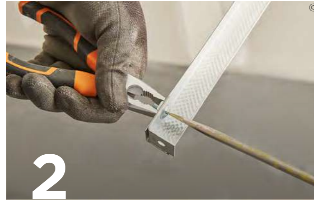
2 Form hangers by securing Gypframe FEA1 Steel Angle or Gypframe MF8 Strap Hanger to Gypframe MF12 Soffit Cleats with Gypframe MF11 Nuts and Bolts.
