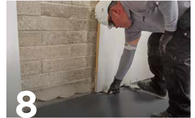
8 Lift boards tight to the ceiling using a foot lifter and support until the adhesive sets.
