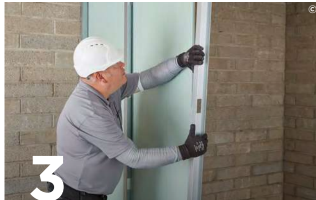
3 Friction fit Gypframe 'I' Studs or Gypframe Tabbed 'I' Studs into the channels at 600 mm required centres. Fit Gyproc CoreBoard or 20 mm Glasroc F FireCase between the studs on the shaft side.
