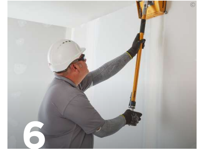
6 Mechanical jointing tools can be used as an alternative to hand jointing, to provide a fast, consistent finish using the bazooka for tape application and the 175mm, 250mm and 300mm finishing boxes as appropriate sanding and decoration preparation remains the same.
