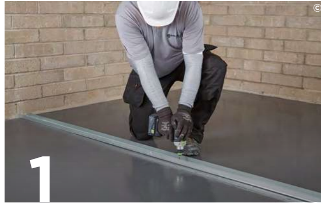
1 Suitably fix the appropriate Gypframe floor and ceiling channels to the perimeter at the required centres.
