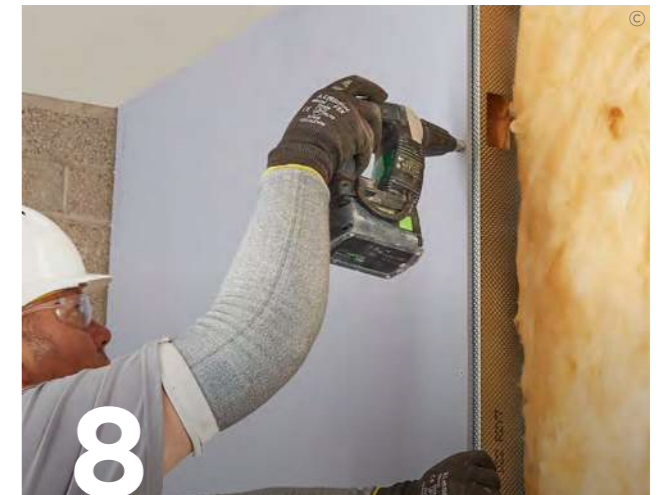
Use British Gypsum Jack-Point Screws to fix Gyproc SoundBloc plasterboards to alternate Gypframe 'I' Studs and other framing members.
