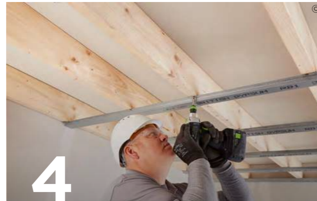
4 Use British Gypsum Drywall Screws to install Gypframe RB1 Resilient Bars to the underside of the joists.
