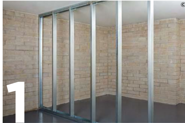
1 Completed Steel Framing System (SFS) framework ready to receive the Glasroc X Sheathing Board.
