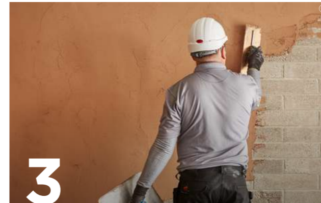
3 Select the correct Thistle plaster to suit the background suction and surface texture. Apply the plaster in maximum 8mm coats. Allow each coat to set before applying the next.
