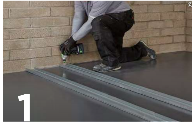
1 Suitably fix the appropriate Gypframe Floor & Ceiling Channels at the required centres to the floor and soffit.
