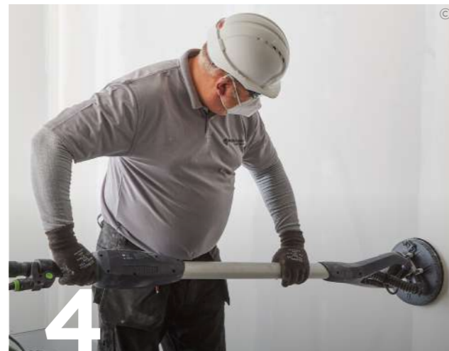
4 Once dried, the joint treatment is sanded as necessary to achieve a smooth surface.
