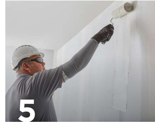
5 Gyproc Drywall Primer or Gyproc Drywall Sealer is applied to the entire board surface and jointed areas, to control suction and prepare the lining for final decorative treatment.
