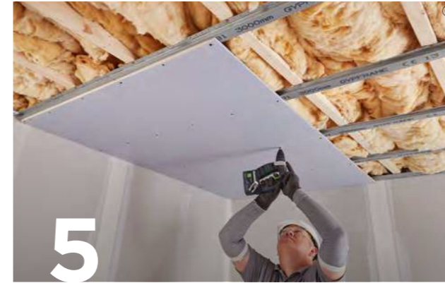
5 Lay 100 mm Isover Spacesaver Ready-Cut between joists and rest on the Gypframe RB1 Resilient Bars. Use British Gypsum Drywall Screws to fix the specified ceiling board fixed to the Gypframe RB1 Resilient Bars.
