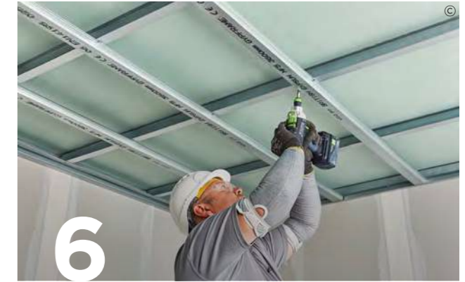
6 Run and fix Gypframe MF5 Ceiling Sections perpendicular to 'I' Studs using appropriate fixings.
