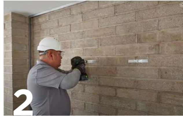
2 Mark vertical lines on the wall at 600 mm intervals to indicate Gypframe GL2 or GL9 Bracket fixing centres. Mark horizontal lines at 800 mm centres to determine individual bracket positions. Suitably fix Gypframe GL2 or GL9 Brackets into position. Gypframe GL2 or GL9 Brackets should be fixed with Gypframe GL11 GypLyner Anchor.
