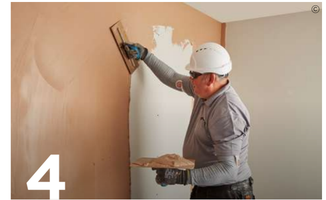
4 Thistle plaster is applied with firm pressure, built out to the required thickness in two applications and trowelled to a smooth matt finish. When applying ThistlePro FastSet Finish, a single mix for both first and second coat is recommended.
