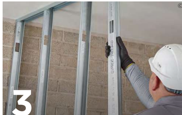
Friction fit Gypframe 'C' studs into the appropriate Gypframe Channels at required centres.
