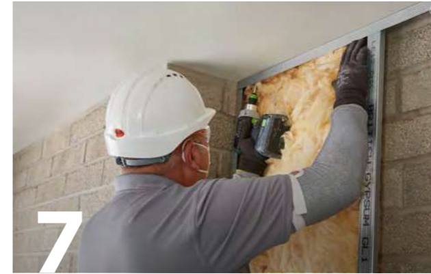
7 Add Isover Acoustic Partition Roll (APR 1200) insulation to the partition cavity for optimal acoustic and thermal performance.
