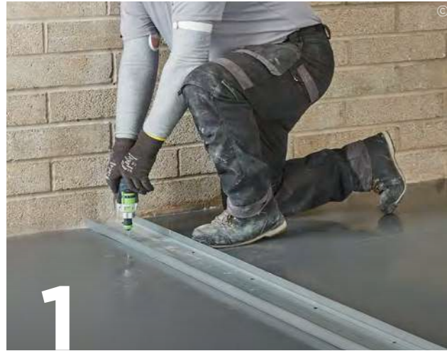
Suitably fix the appropriate Gypframe Floor & Ceiling Channels at the required centres to the floor and soffit.
