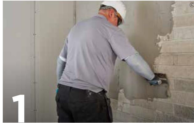
1 Apply Gyproc SoundCoat Plus in a continuous 6mm coat to the entire surface of the external or separating walls for optimum air tightness and acoustics. Allow Gyproc SoundCoat Plus to set before applying of DriLyner Dab using Gyproc DriWall Adhesive.
