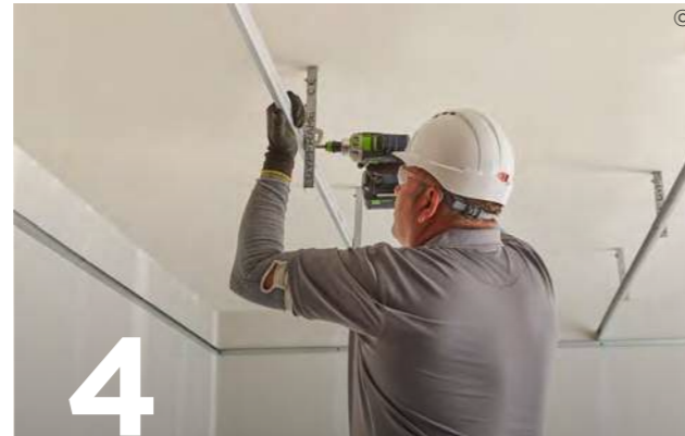
4 Position Gypframe MF7 Primary Support Channels then use British Gypsum Wafer Head Jack-Point screws to fix the hangers to the side of these channels. Use two screws per hanger.
