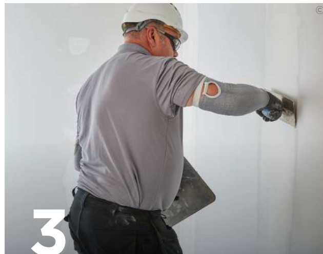
3 Two or three further applications of jointing compound are trowel applied, each feathered out beyond the previous application. An equal number of applications are made to spot screw heads.
