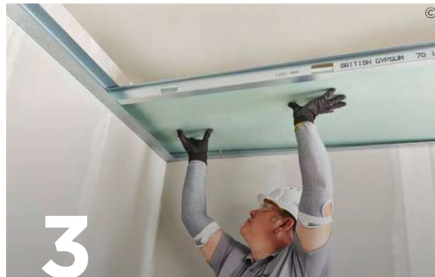
3 Friction fit Gypframe 'I' Studs or Gypframe Tabbed 'I' Studs into the channels at 600 mm required centres. Fit Gyproc CoreBoard or 20 mm Glasroc F FireCase between the studs on the shaft side.
