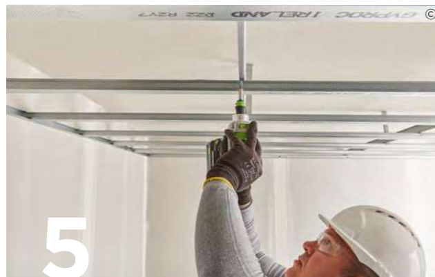
5 Use British Gypsum Wafer Head Jack-Point Screws to fix Gypframe MF5 Ceiling Sections to the underside of the Gypframe MF7 Primary support at required centres.
