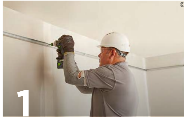
1 Fix Gypframe MF6 Perimeter Channels to the perimeter walls at 600 mm centres.
