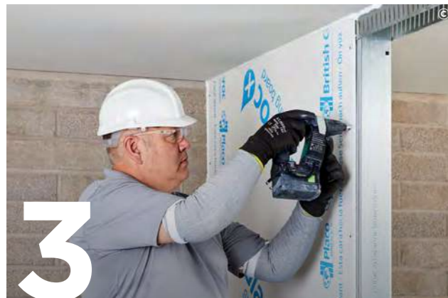
3 Use Glasroc X Screws 25 mm to fix Glasroc X Sheathing Board to the SFS framework.
