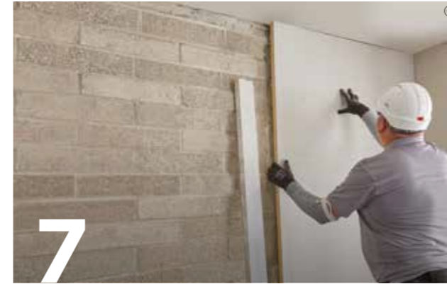
7 Offer up boards and tap into position. Be careful to avoid creating wave and hollows.
