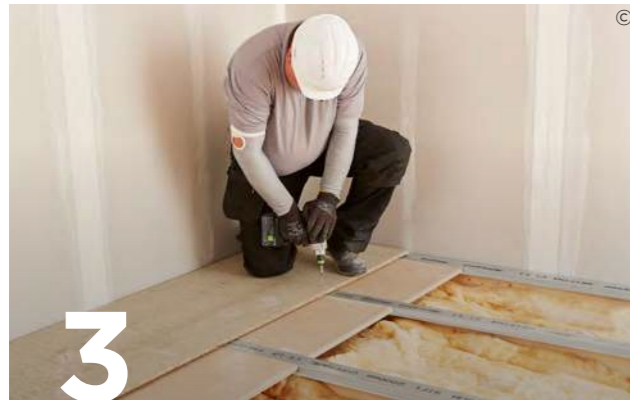
3 Lay flooring across the Gypframe SIF Floor Channels. Use Gypframe SIF5 Floor Screws to fix through the Gyproc Plank to the channel flange on one side only.
