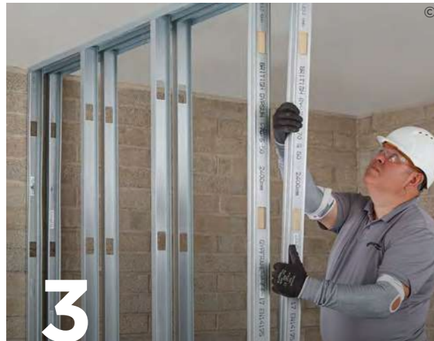
3 Friction fit Gypframe 'I' Studs into the appropriate Gypframe Floor & Ceiling Channels at the required centres.
