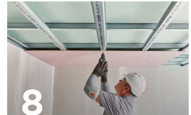
8 Gyproc plasterboards are then fixed to the Gypframe framework with British Gypsum Drywall Screws to metal framing less than 0.8 mm thick ('I' Studs less than 0.6 mm thick) or British Gypsum Jack-Point Screws to metal framing 0.8 mm thick and greater ('I' studs 0.6 mm thick and greater).
