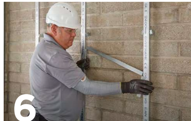
6 Construct door and window openings with Gypframe GL8 cut and bent to form the head of the opening and fix to the side of the channel using two British Gypsum Wafer Head Drywall Screws
