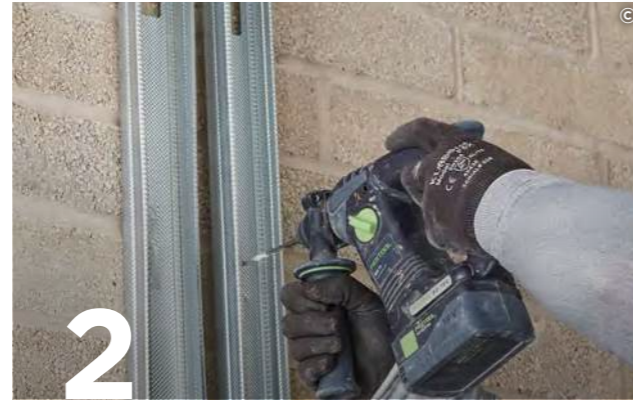
Fix Gypframe 'C' Studs at abutments and openings in two rows using suitable fixings.
