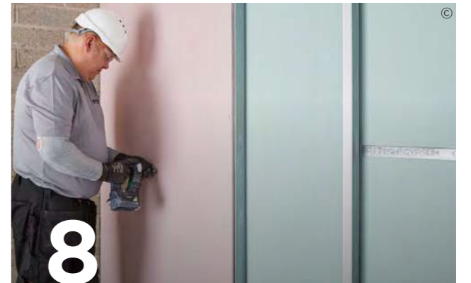
8 Gyproc plasterboard or Glasroc F FireCase are then fixed to the Gypframe framework with British Gypsum Drywall Screws to metal framing less than 0.8 mm thick ('I' Studs less than 0.6 mm thick) or British Gypsum Jack-Point Screws to metal framing 0.8 mm thick and greater ('I' studs 0.6 mm thick and greater).
