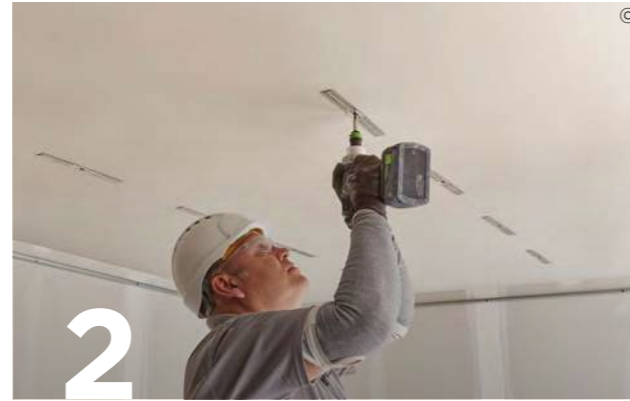
2 Suitably fix Gypframe GL2, GL9 or GL12 Brackets as required to the soffit at the required centres.
