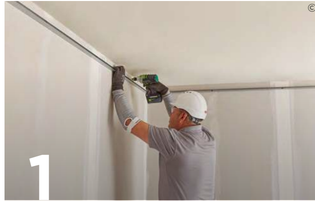
1 Suitably fix Gypframe GL8 Perimeter Channels to the perimeter walls at the required centres. Ensure the large lip is positioned at the bottom.
