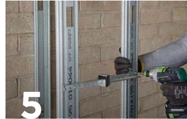
5 Brace the Gypframe 92 S 10 'C' Studs together in pairs. Brace with either a staggered Gypframe GAB3 Acoustic Brace or a Gypframe 99 FC 50 Fixing Channel. For Gypframe GAB3 Acoustic Braces fix at 3300 mm centres with two British Gypsum Wafer Head Drywall Screws. For 99 FEC 50 fix at 3600 mm centres with four British Gypsum Wafer Head Drywall Screws.
